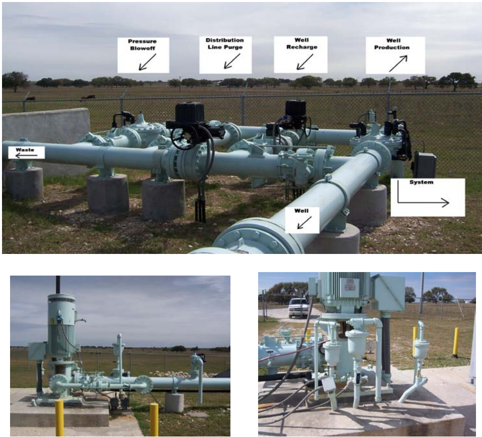
Figure 5: Well Equipping (Morris, 2006)
