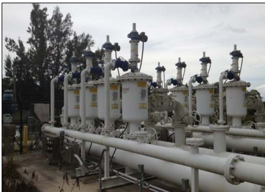
Figure 6-15 -- Amiad filtration system.
