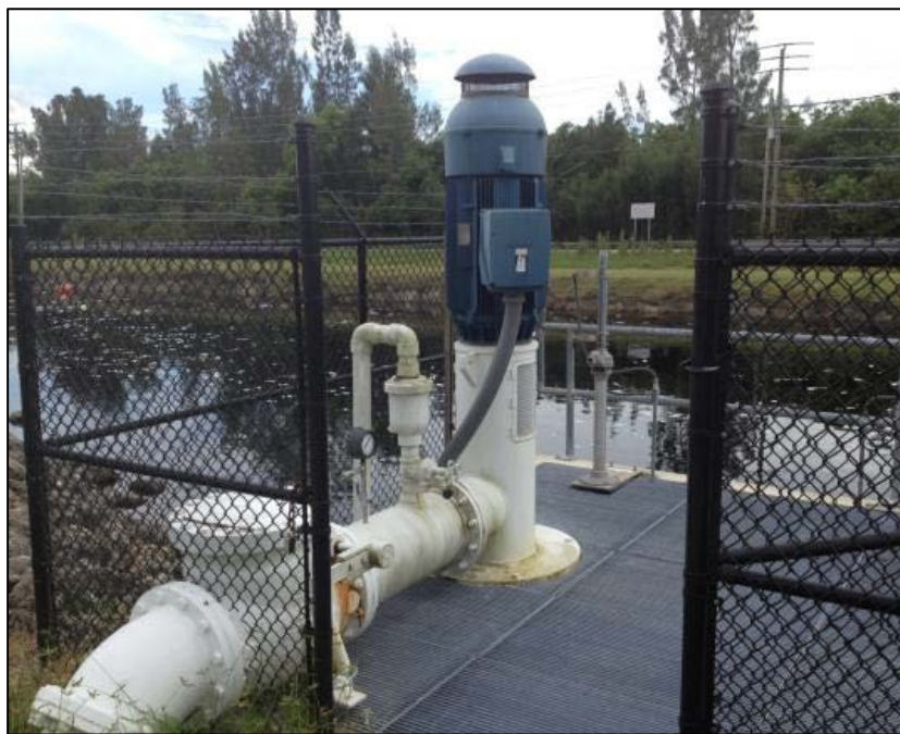
Figure 6-14 -- Recharge pump at the intake structure.
