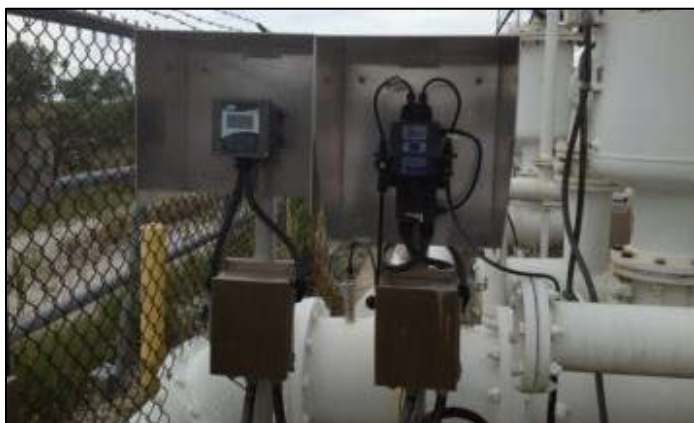
Figure 6-19 -- Water quality monitoring components.
