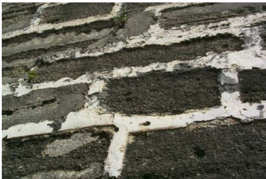
Figure 9. Erosion of surface of coquina stones. (Photo courtesy of the author.)
