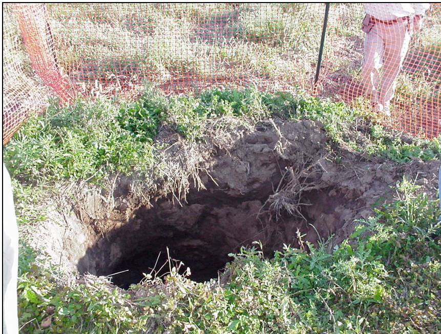
Figure 7-7 Sinkhole near Lexington, KY
