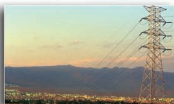
Electric tower, Mexico.
