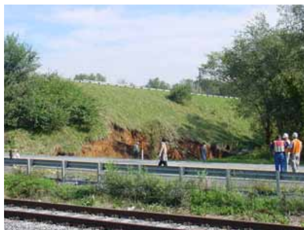
Figure 3. Cover-collapse sinkhole due to changed subsurface drainage conditions. Note proximity of railway to sinkhole
