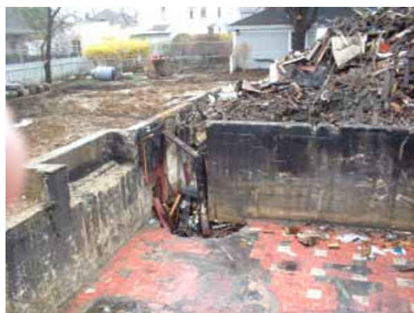
Figure 2. Sinkhole that compromised existing foundation.
