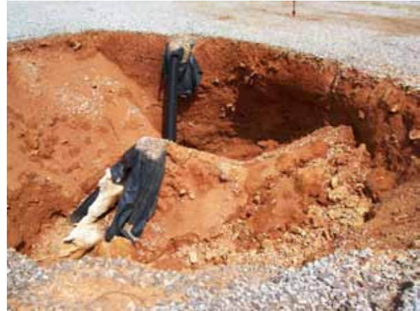
Figure 6. Sinkhole development as a result of concentrated surface water
