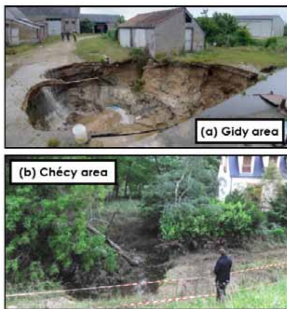
Figure 4. Two major sinkholes triggered by floods.
