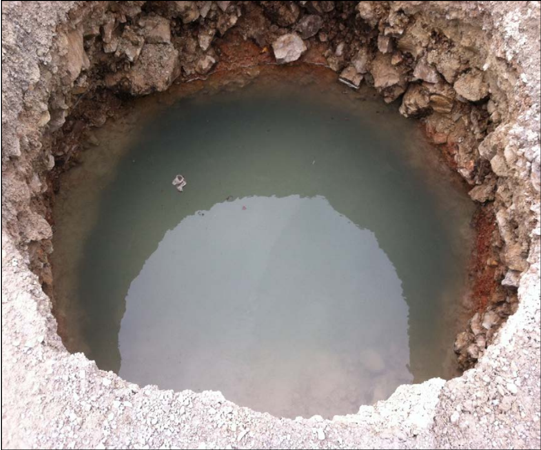
Figure 8.2. Mapped Sinkhole in the parking lot
