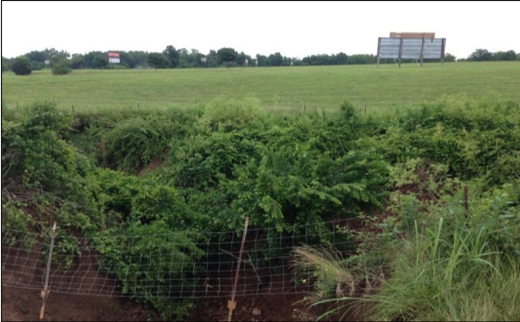
Figure 6.2. Sinkhole in the project site covered with barrier for safety purpose
