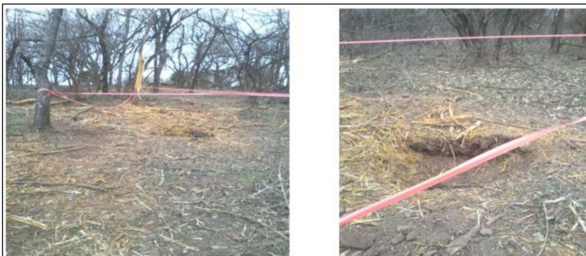
Figure 10.2. Sinkhole development in the area starting with soil depression
