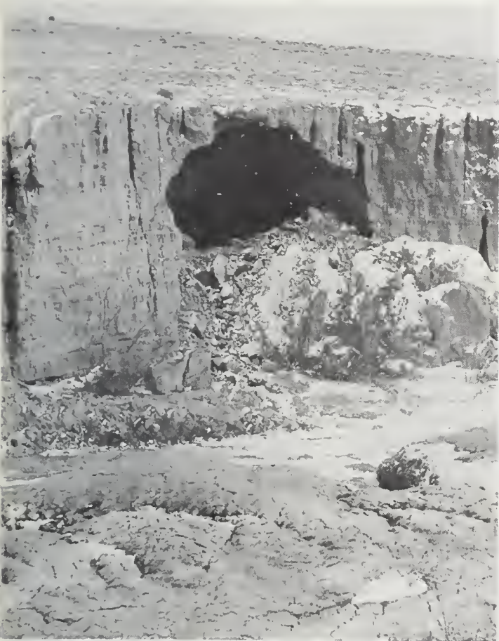
FIGURE 14. — Soil pipe openings on a side slope and in a gully wall representing the pipe inlet and outlet.
