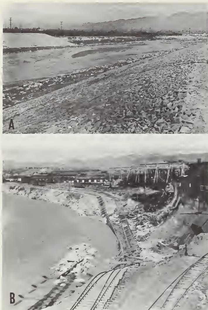
FIGURE 6.—Upstream views of Los Angeles River channel after 1938 flood: A , Right bank destroyed downstream from Verdugo Wash confluence; B , left bank damaged along outside of bend.
