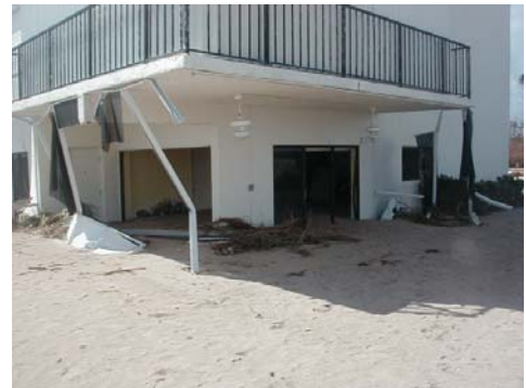
Properties with insufficient setbacks from the ocean are prone to extensive storm surge damage.
