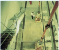
Huge master lift stations are more than thirty feet underground.
