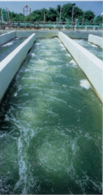
Water runs through the advanced secondary treatment process...at the end the final product looks like swimming pool water.
