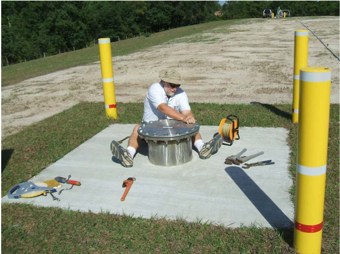
Figure 8. Final wellhead, POF-29.
