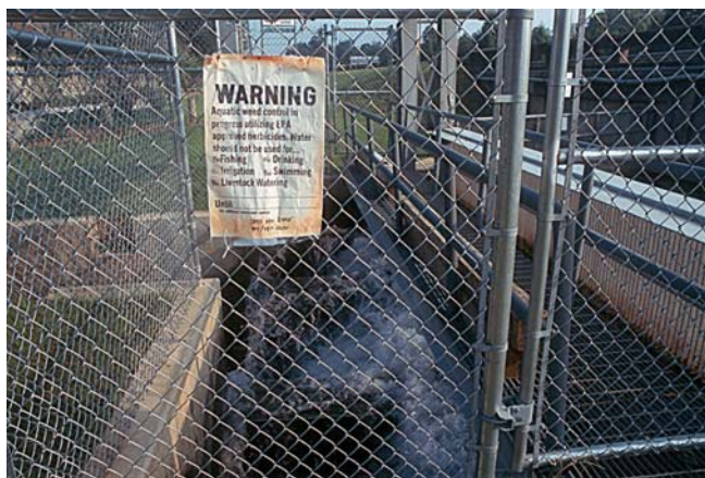
Figure 5. Weir prevented plant material from flowing downstream. Photo taken 7/97 by Carl R. Froede Jr.
