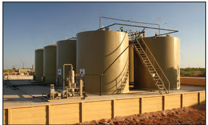
Secondary containment structure-
