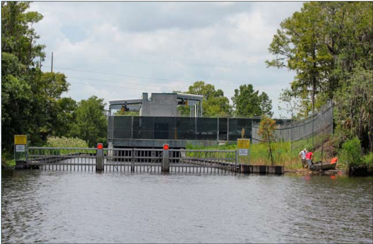
Seminole County intake – Seminole County withdrawal structure on middle St. Johns River. Photo / Gary Raulerson
