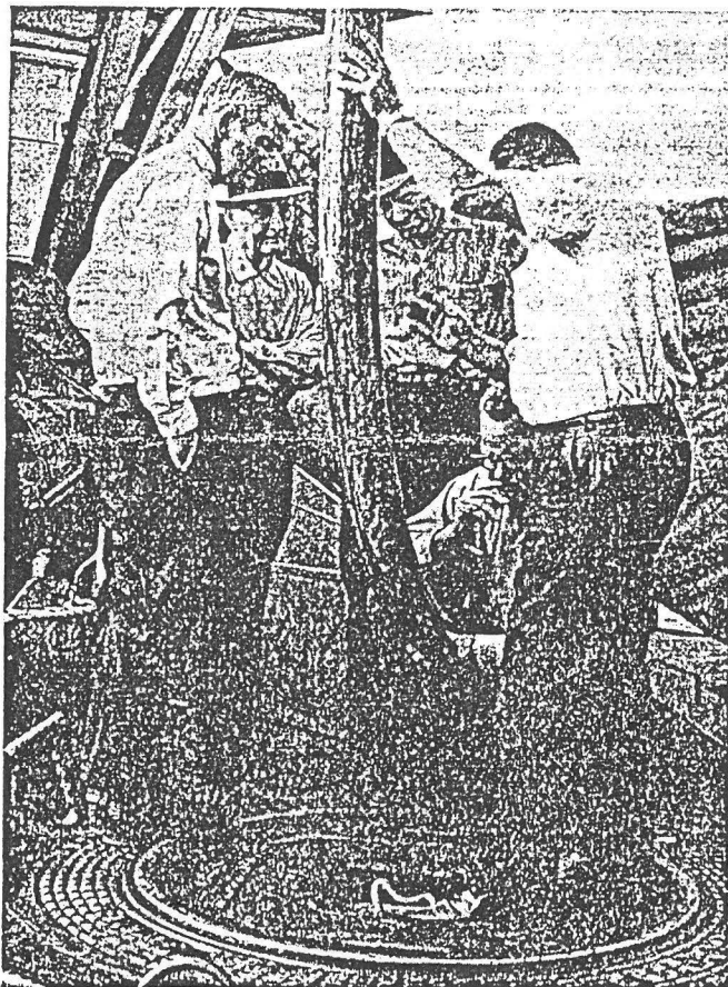
BENT PIPE at troublesome well in Sunoco field shows extent of drilling problems. This drill pipe, pulled from the hole at Sun Oil Co.'s 32-2 Red Cattle Co., was twisted while trying to drill through a 90-ft cavern.
