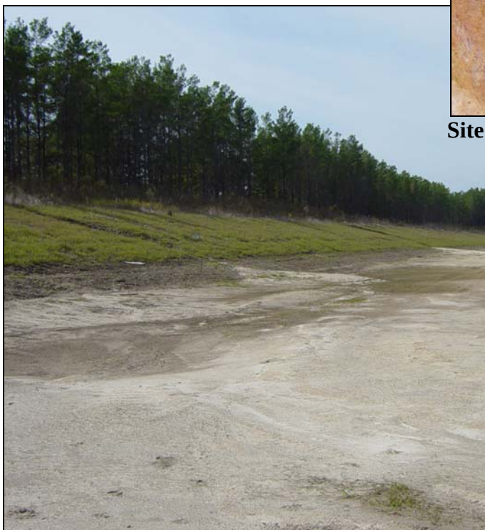
Site 2: Additional depressions forming in Eastern Pond
