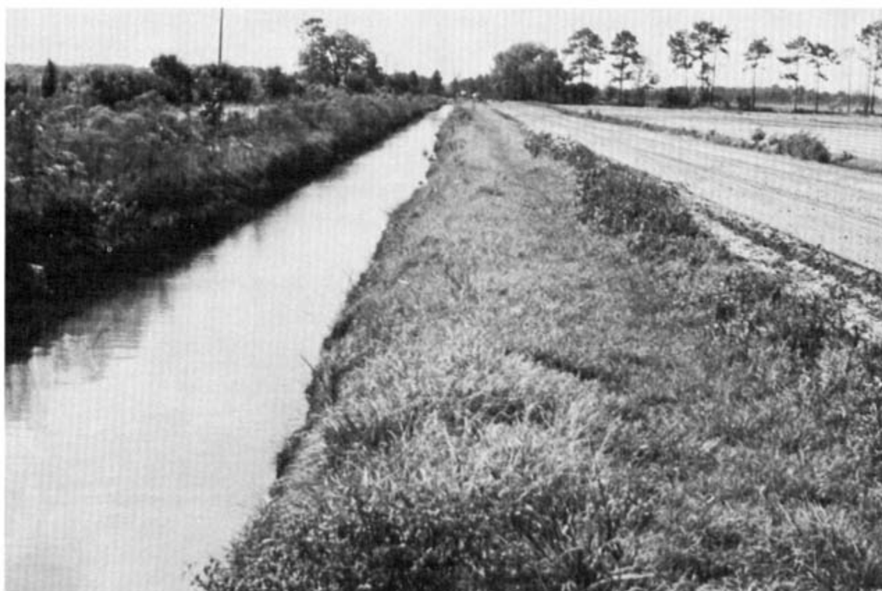
Figure 11. —Water control ditch used for drainage and subsurface irrigation on Smyrna fine sand.
