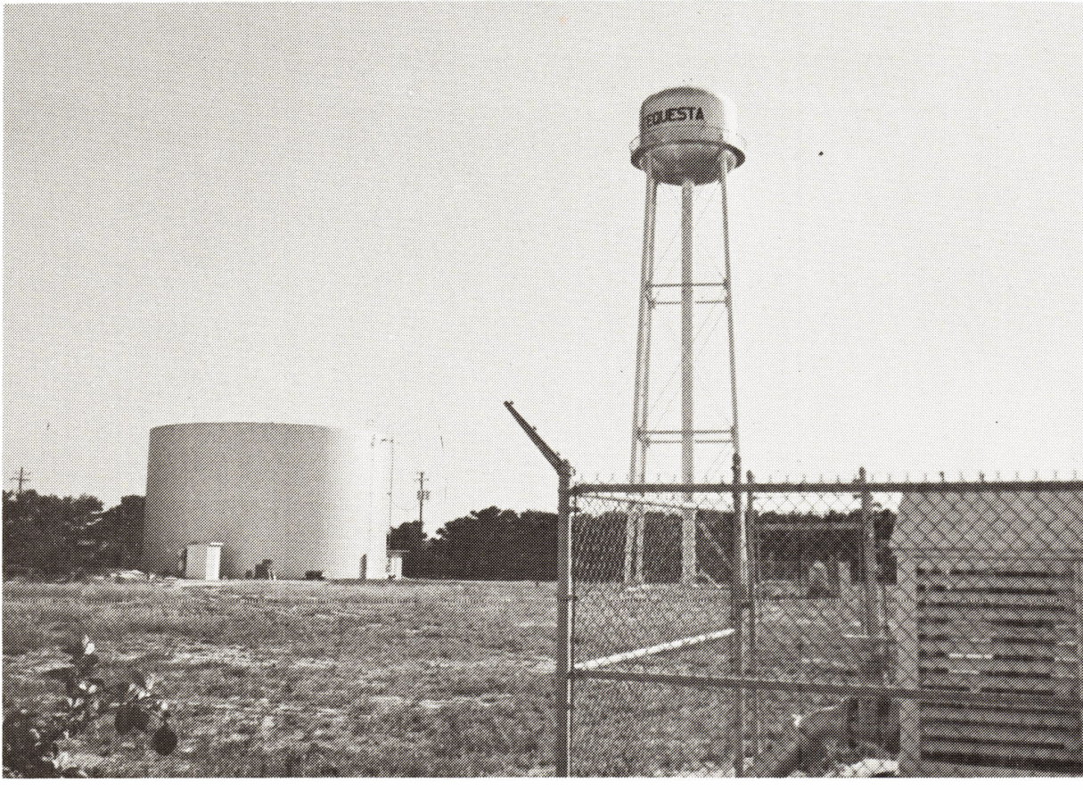
Wells in Tequesta Well Field "1" shown above are 60 to 70 feet deep and yield approximately 500 gallons per minute. Other wells nearby range in depth from 30 to 180 feet and may yield from 5 to 750 gallons per minute. The water is generally of good chemical quality, low in hardness, and low in chloride except where contaminated by adjacent salty-water bodies. Below 180 feet, water becomes scarce and generally is very salty.
