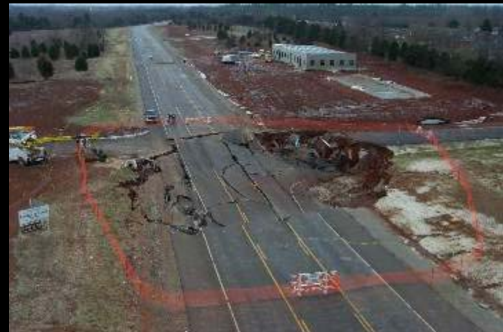
Dishman Lane sinkhole collapse, Bowling Green, Kentucky – Photo Center for Cave and Karst Studies, Western Kentucky Univ.
