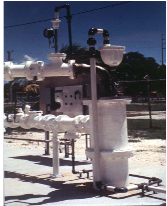
Marathon ASR, Florida (Not in current operation. First ASR well to successfully store drinking water in a seawater aquifer.)
