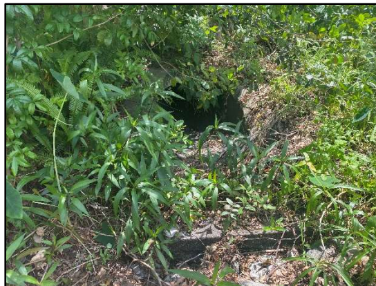
2390, mitered end section at outfall BLA3, looking south toward Raeford Rd.
