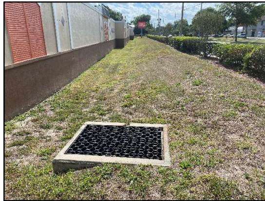
2316, grated drop inlet in retention pond on north side of Michigan St., looking east
