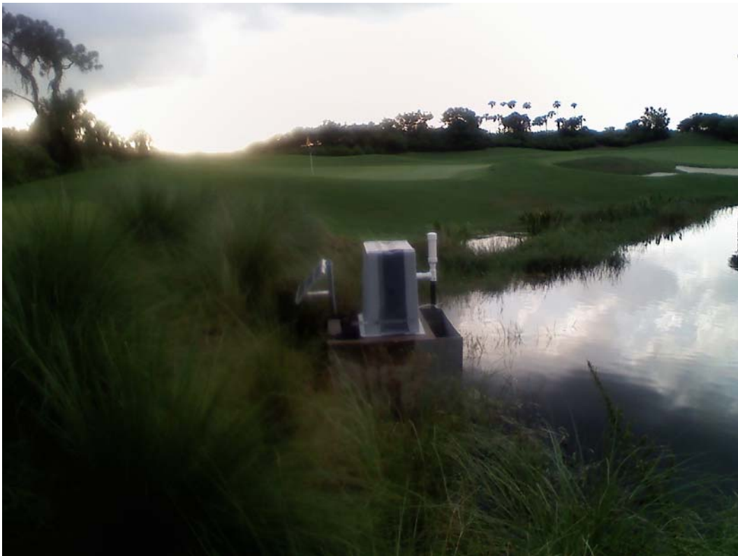
Verandah L29 outfall and Avalanche sampler.
