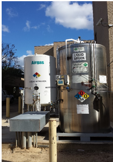
Figure 11.4 Bulk Nitrogen & Argon Tank
