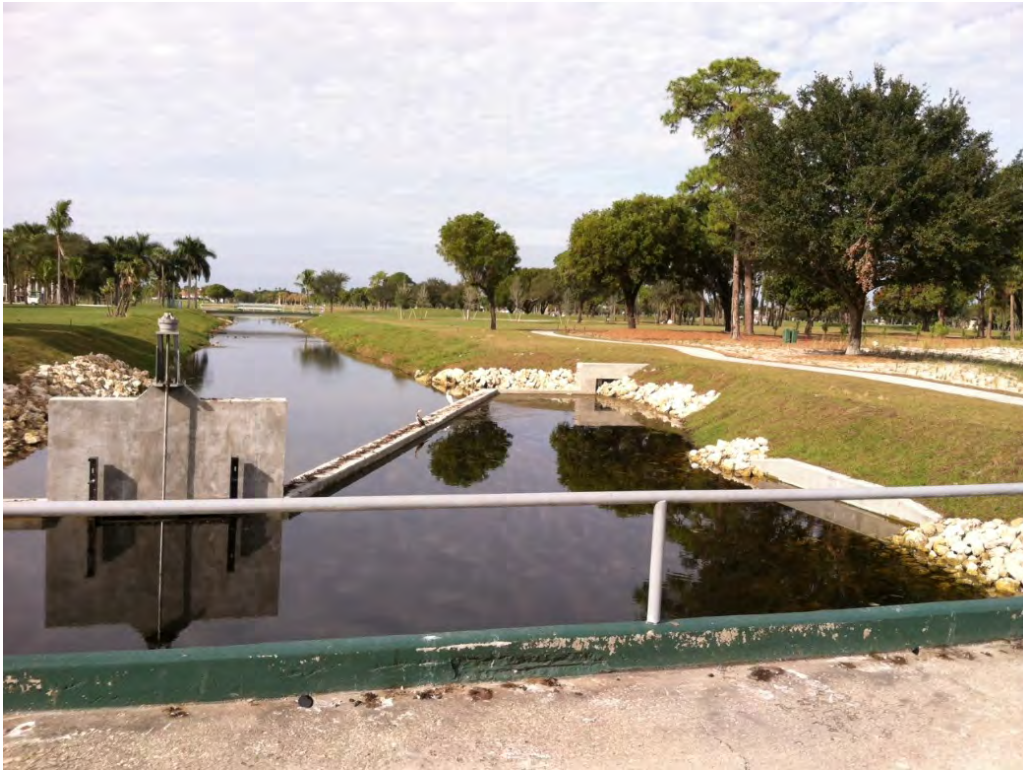
FIGURE 3: CITY OF FORT MYERS CARRELL CANAL WATER QUALITY RETROFIT
