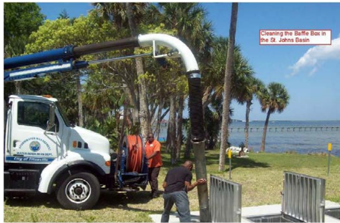
FIGURE 13: CITY OF TITUSVILLE BAFFLE BOX CLEAN OUT
