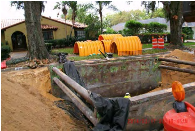
FIGURE 7: CITY OF WINTER PARK NORTH EXFILTRATION TREATMENT PROJECT
