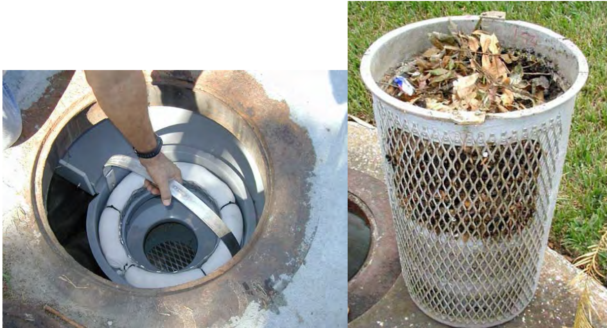
FIGURE 9: ORANGE COUNTY CLEAN INLET BASKET INSIDE CURB INLET (LEFT) AND INLET BASKET FULL OF DEBRIS READY FOR PROCESSING (RIGHT)
