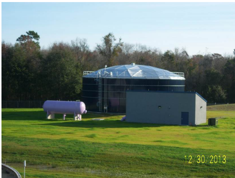
FIGURE 7: CUA NEW RECLAIMED WATER STORAGE TANK AND PUMPING STATION AT RIDAUGHT LANDING WWTF
