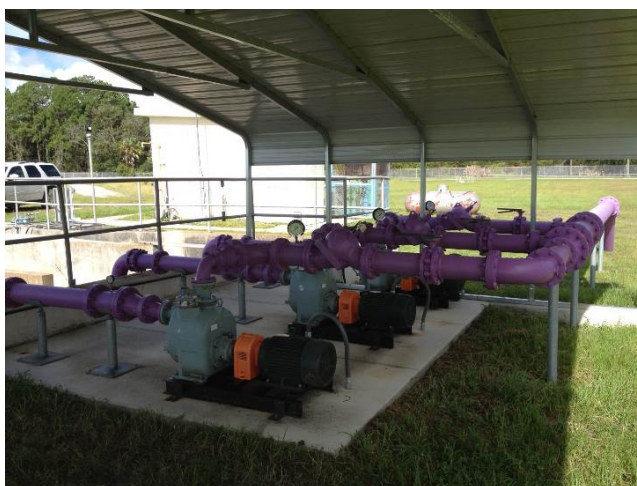
FIGURE 10: NAS JACKSONVILLE REUSE PUMP STATION AT THE WWTF
