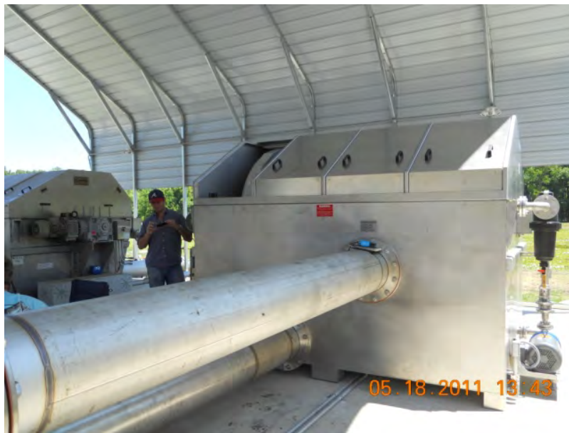
TERTIARY FILTER #2 AT THE ASH STREET WWTF
