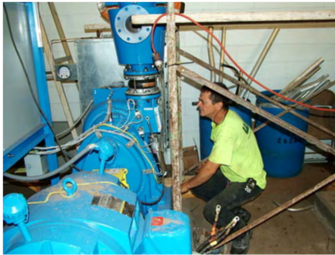
INSTALLED MORE EFFICIENT BLOWERS
