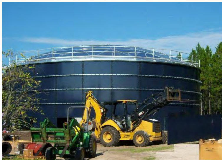
FIGURE 17: CCUA NEW 0.75 MILLION GALLON GROUND STORAGE TANK AT OAK LEAF PLANTATION
