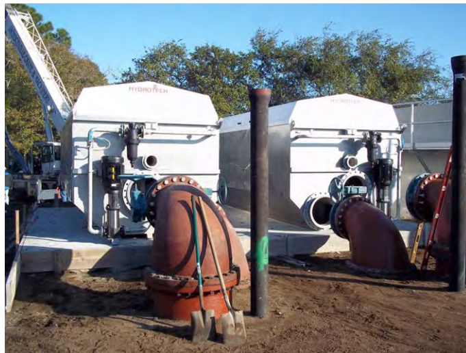
EFFLUENT FILTERS INSTALLED AT WWTP #1
