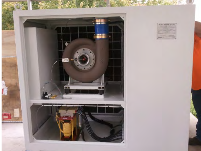
ASH STREET WWTF NEUROS TURBINE BLOWERS
