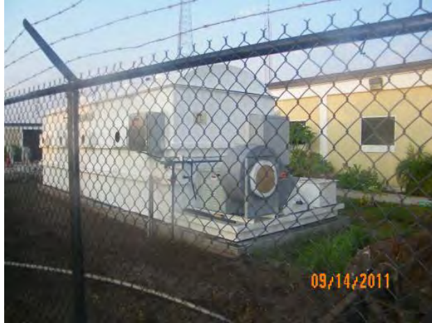
FIGURE 11: JACKSONVILLE BEACH WWTP NEW ODOR CONTROL EQUIPMENT
