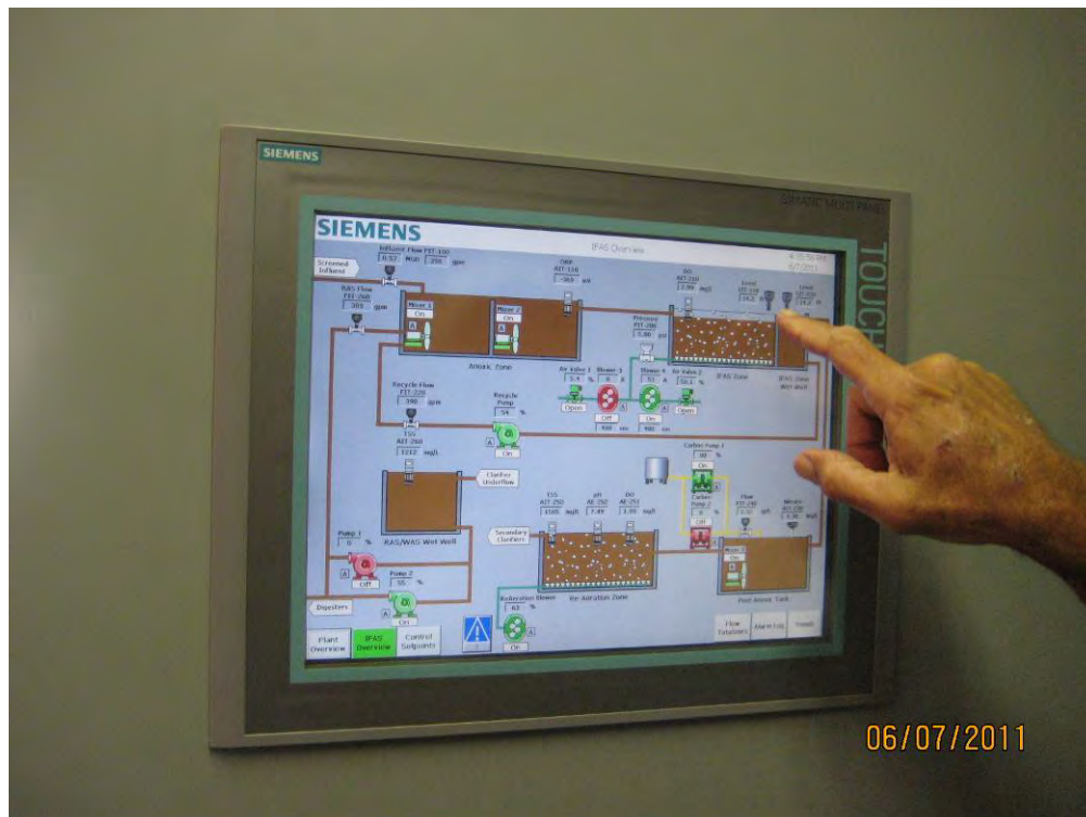
CONTROL PANEL FOR THE NEW NEPTUNE BEACH WWTf
