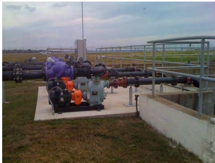
FIGURE 22: NEW REUSE PUMPS FOR PHASE 1 EXPANSION AT NAS JACKSONVILLE
