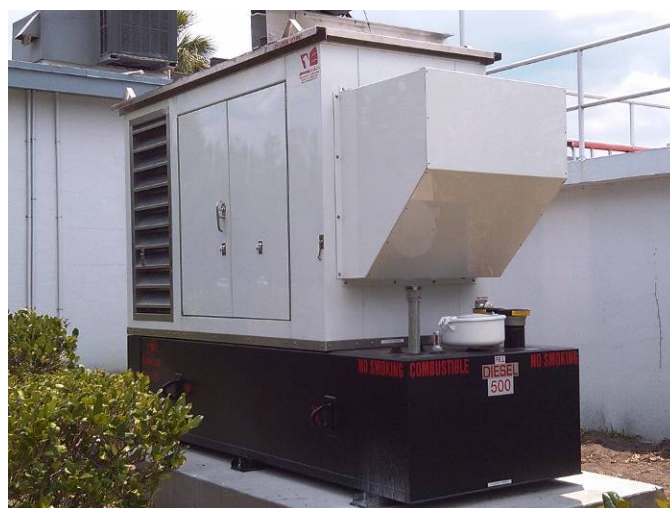
NEW 100 KILOWATT GENSET REPLACED OLD 300 KILOWATT GENSET
