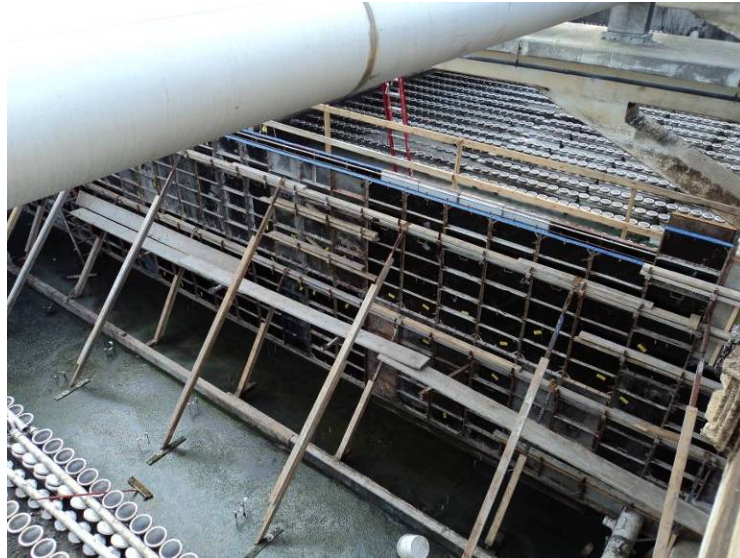
FIGURE 11: JEA UPGRADES AT THE BUCKMAN WWTF
