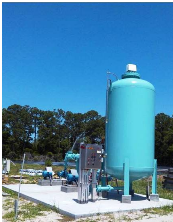
ON-SITE REUSE SYSTEM INSTALLED FOR WATER CONSERVATION
