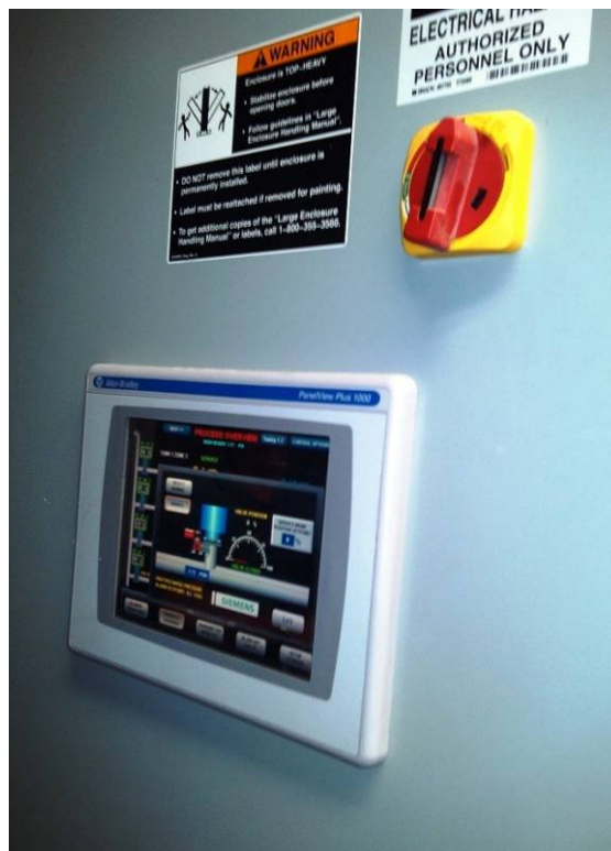
PROGRAMMABLE BLOWER SETTINGS PROVIDE PLANT OPERATORS WITH FLEXIBILITY
