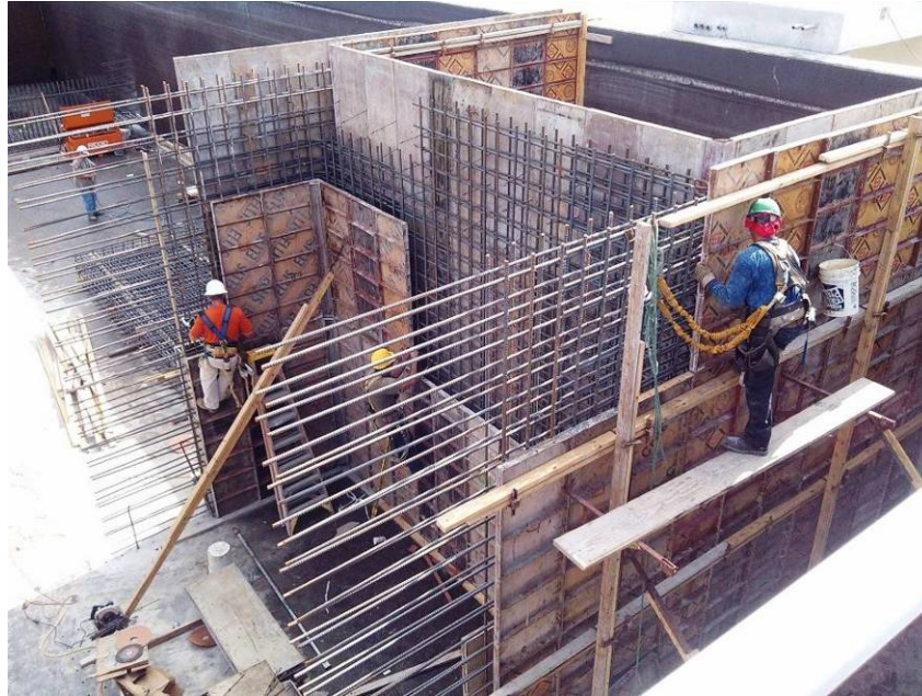
FIGURE 7: CITY OF ATLANTIC BEACH EXISTING WWTP #1 TANKAGE MODIFIED TO PROVIDE 4-STAGE NITROGEN REMOVAL PROCESS
