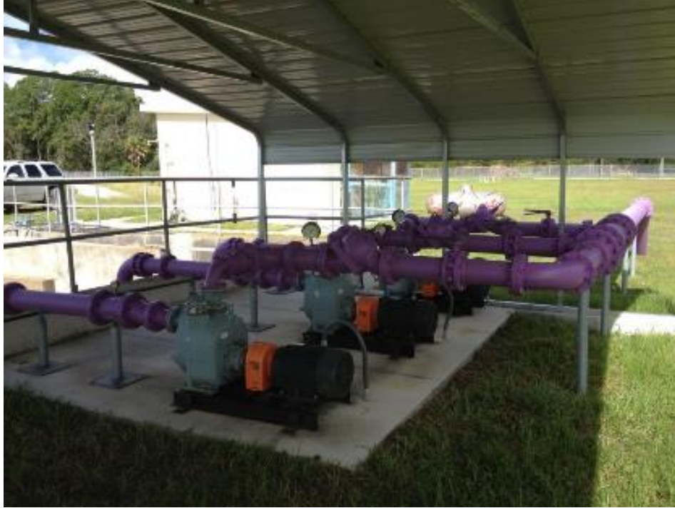
FIGURE 6: NAS JACKSONVILLE REUSE PUMP STATION
