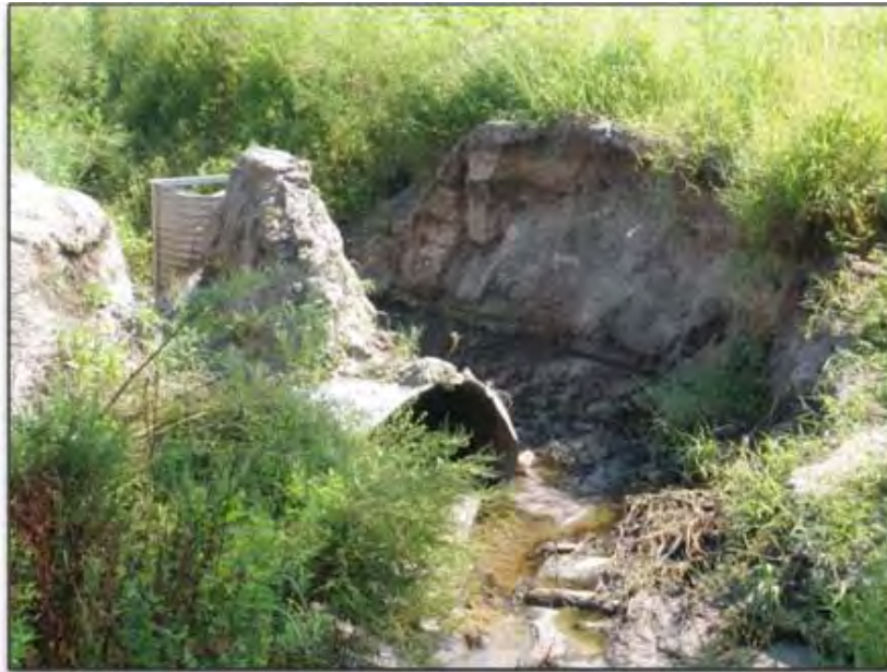
BLOWN-OUT CULVERT FROM SPRING STORMS
