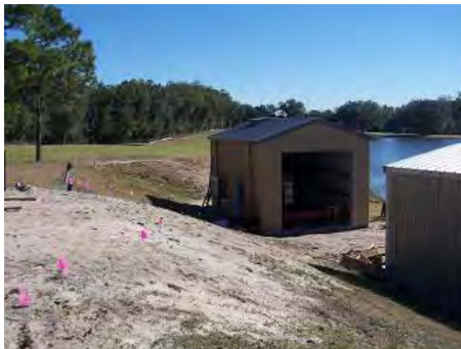
NEW RECLAIMED WATER PUMPING STATION WITH BUILDING
