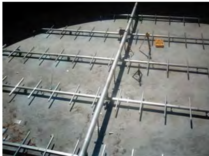
COARSE BUBBLE DIFFUSER ARRAY IN DIGESTER #2
