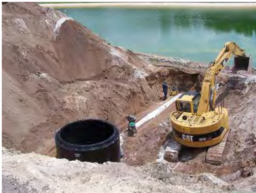
FIGURE 3: CITY OF PALATKA WET WELL PIPE CONNECTION TO RECLAIMED WATER HOLDING POND
