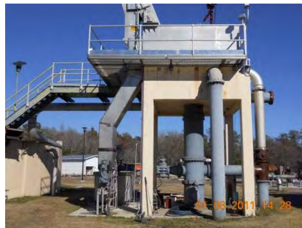
MECHANICAL BARSCREEN AND TRASH COMPACTOR PLACED IN SERVICE ON DECEMBER 7, 2009
