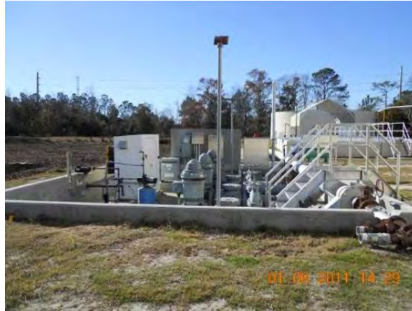
STORMWATER INTRUSION PROBLEM SOLVED
