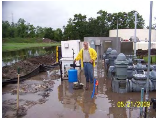
FLOODING FROM STORMWATER POND COMPROMISES EFFLUENT QUALITY
