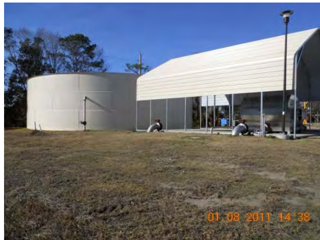
DIGESTER #2 (ON LEFT) AND TERTIARY FILTER #1 (ON RIGHT)
