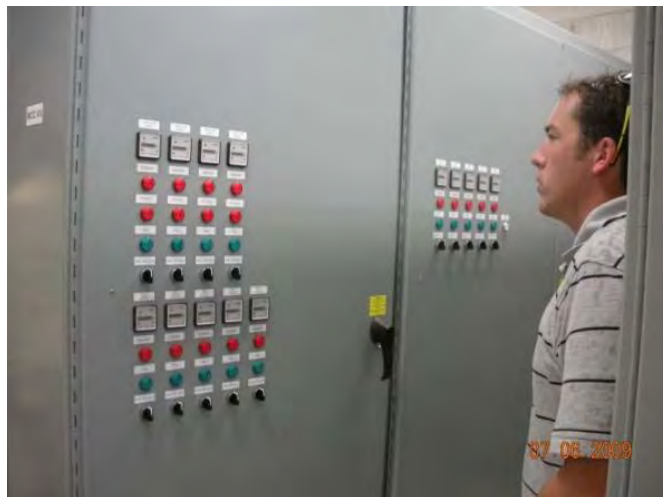
MOTOR CONTROL CENTER
