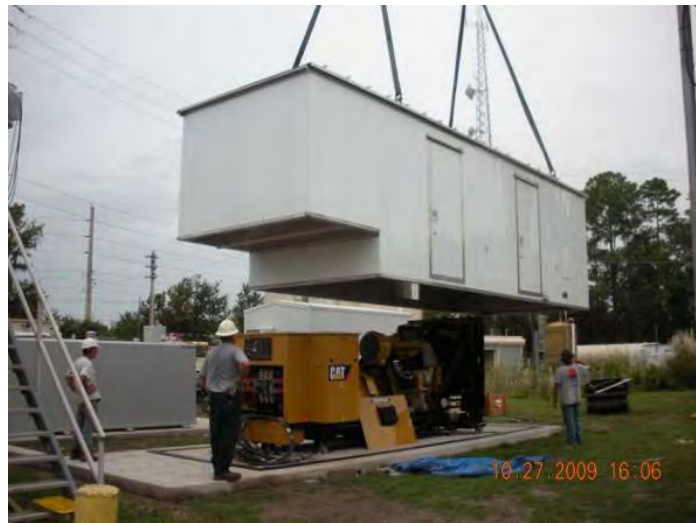
1000 kW EMERGENCY GENERATOR
