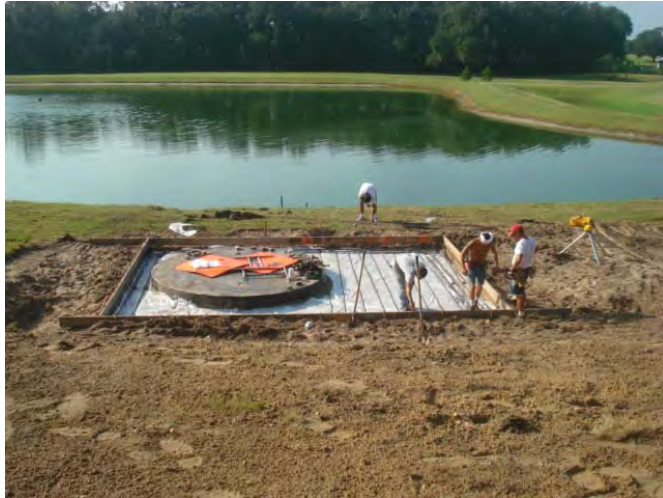
PUMP STATION AT THE GOLF COURSE
