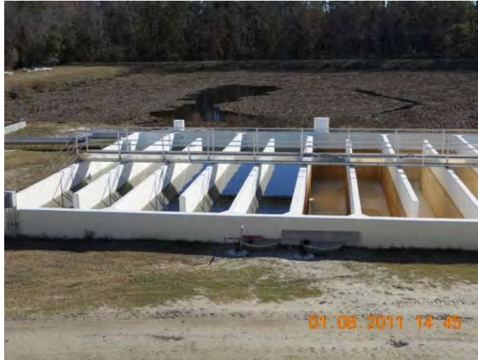
CHLORINE CONTACT CHAMBERS
