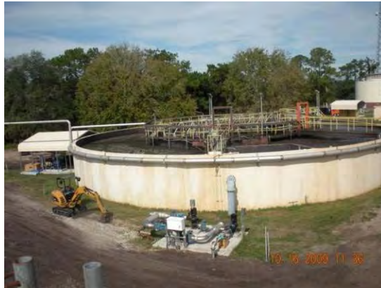
PLANT #3 PRIOR TO BNR CONVERSION
