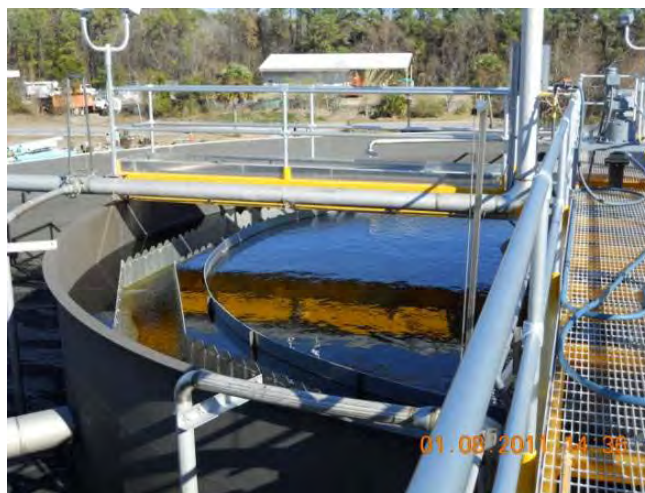
CLARIFIER #4 (INNER RING) AND DIGESTER #1 (OUTER RING)
