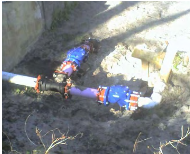
REUSE TIE-IN AT THE RAVINES
