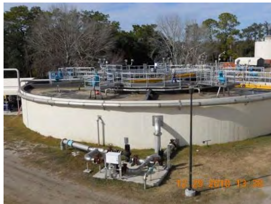
PLANT #3 AFTER BNR CONVERSION (PLACED INTO SERVICE JULY 31, 2010)
