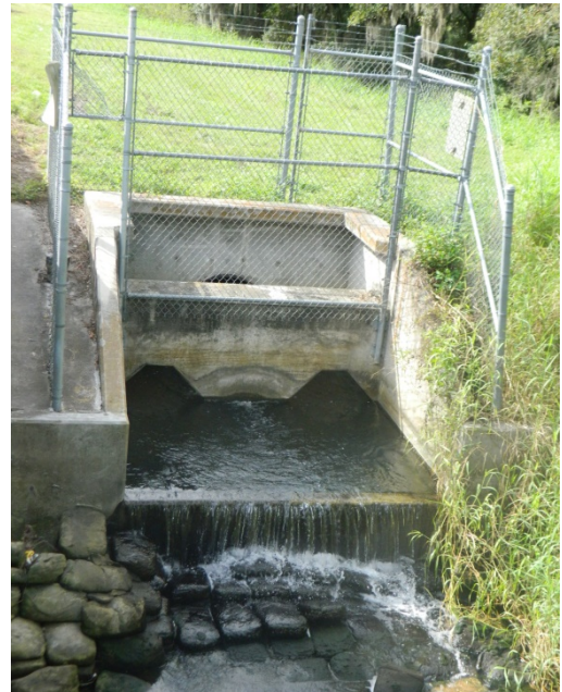
Figure 2. Plant City WRF D-002 outfall to East Canal.
