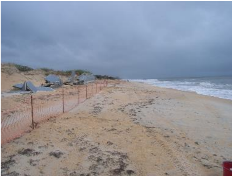
View north from R-50 showing damaged seawall into Varn
