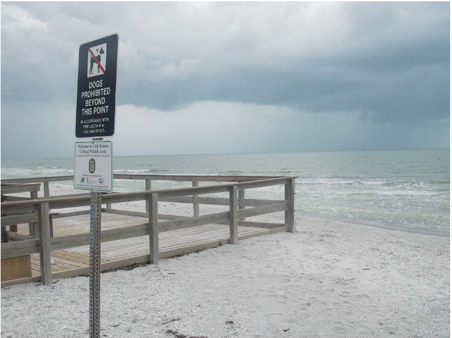
Pier at Leonardo Arms Condo 7400 Estero R-204.5. The pier and condo are now directly exposed to the Gulf rather than the CWA sand bar
