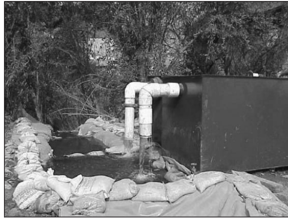
Dewatering tank (Source: http://www.dot.ca.gov )
