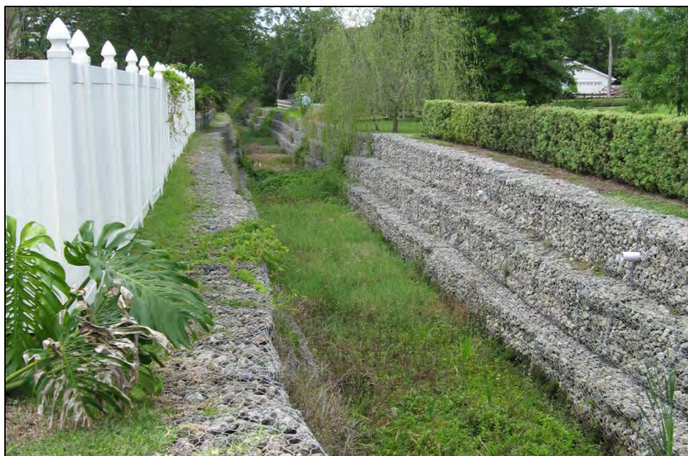
Figure 16. Site P – Coachman Ridge – showing the gabion system and lack of marginal vegetation along Channel F of Alligator Creek.
