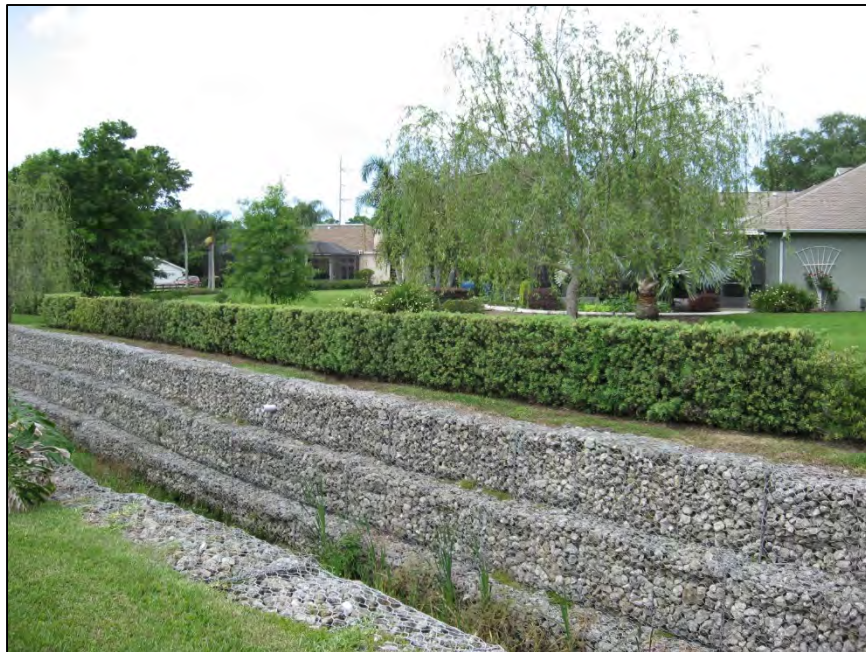
Figure 31. Site P – Coachman Ridge – Roof drains from adjacent residences penetrating the gabion system along Channel F of Alligator Creek.
