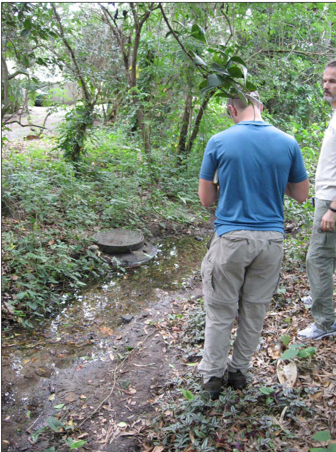
Figure 23. Site M – Sanitary sewer line adjacent to surface water conveyance feature.
