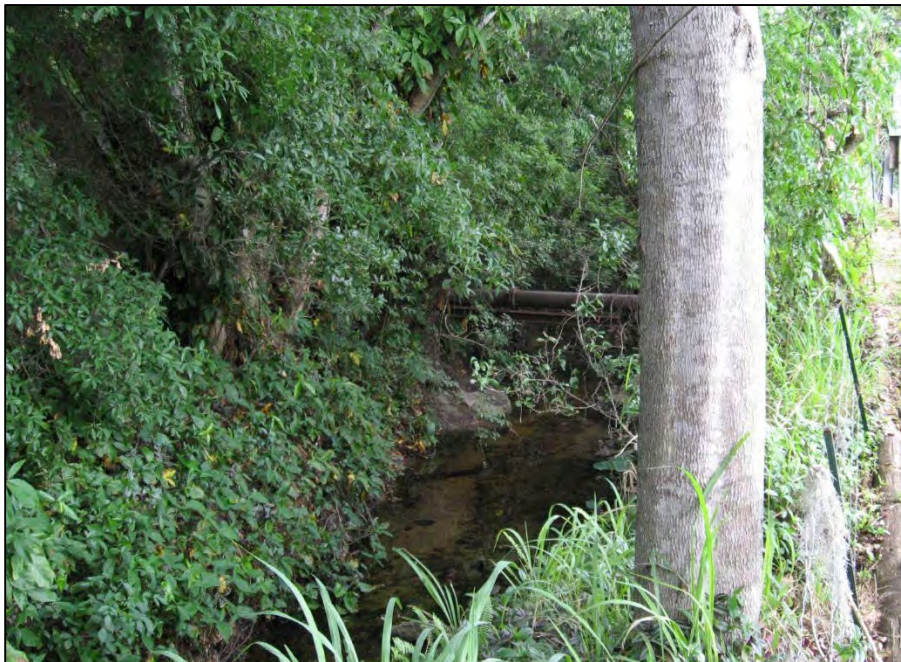
Figure 18. Site F - Alcove Park Mobile Home Park – Aerial crossing of Channel C of Alligator Creek by a ductile iron sanitary sewer pipe.
