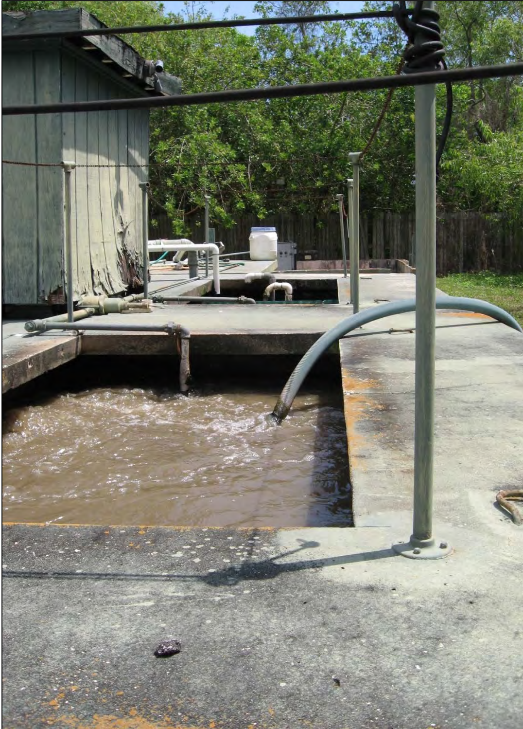
Figure 5. Site A – Southern Comfort Mobile Home Park – Sewage treatment plant adjacent to wetland margins of Alligator Creek (Channel B).
