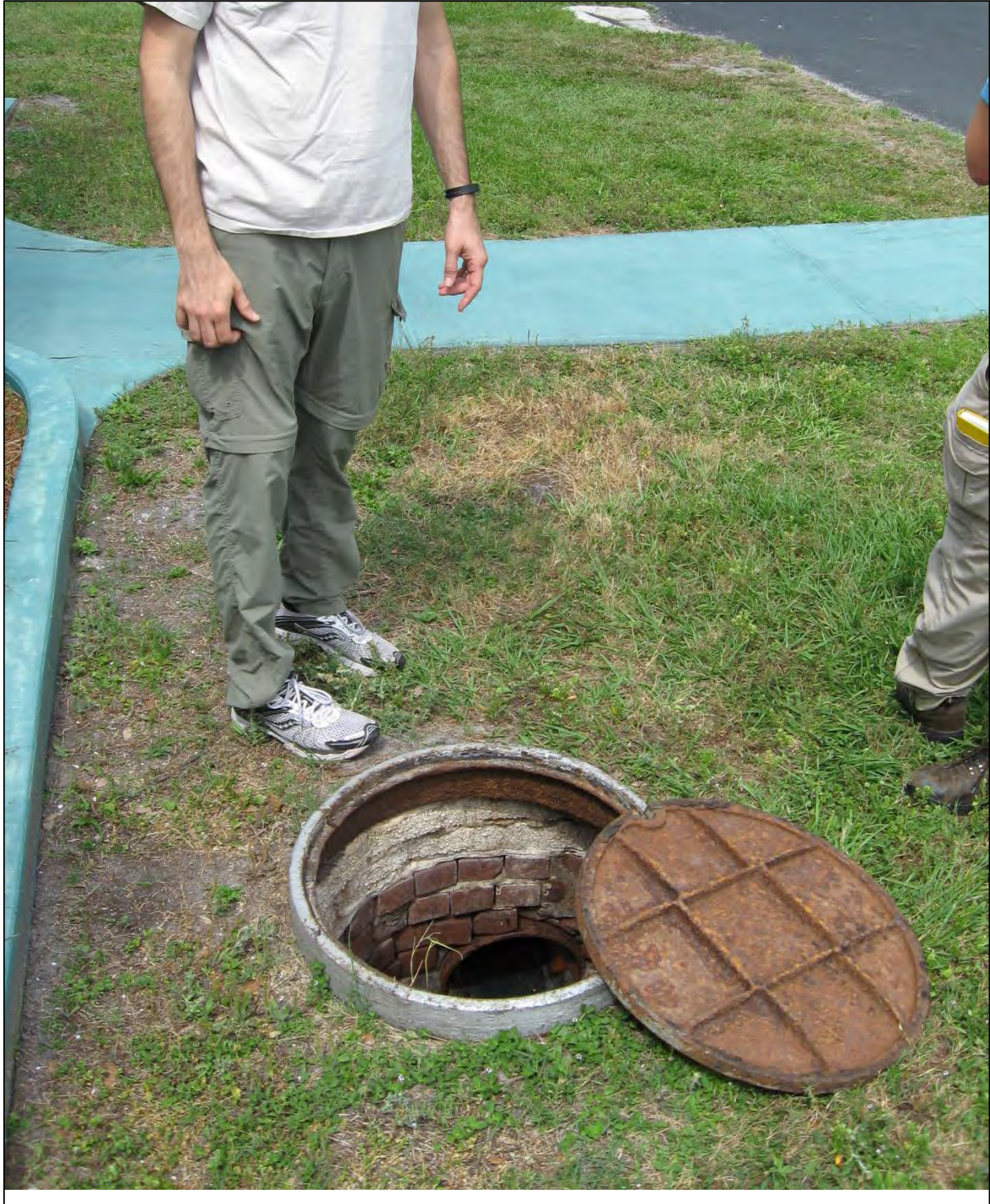
Figure 20. Site F – Alcove Park Mobile Home Park – Sanitary sewer line running from a recreation center within the park toward the ductile iron pipe crossing Channel C of Alligator Creek.
