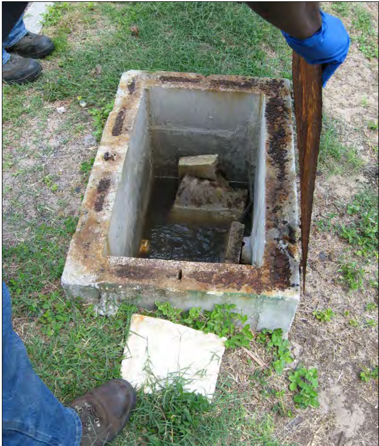
Figure 8. Site A – Southern Comfort Mobile Home Park – Effluent disposal system access is not secured (unlocked).
