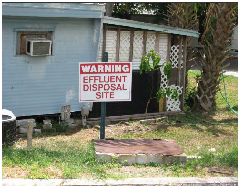
Figure 7. Site A – Southern Comfort Mobile Home Park – Effluent Disposal System. Treated wastewater is pumped up hill to higher areas of the park where it is allowed to infiltrate into the ground.
