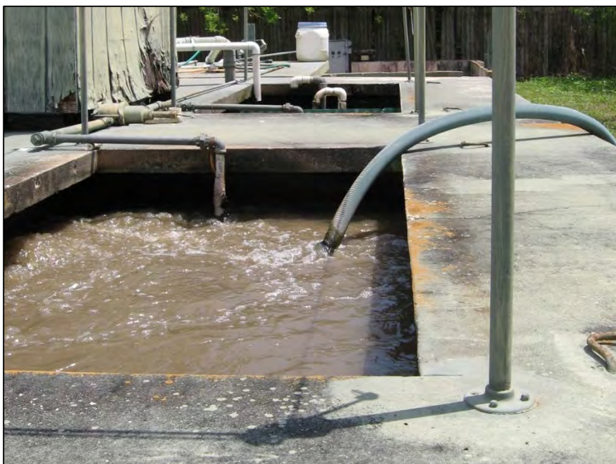
Figure 5. Site A – Southern Comfort Mobile Home Park – Sewage treatment plant adjacent to wetland margins of Alligator Creek (Channel B).
