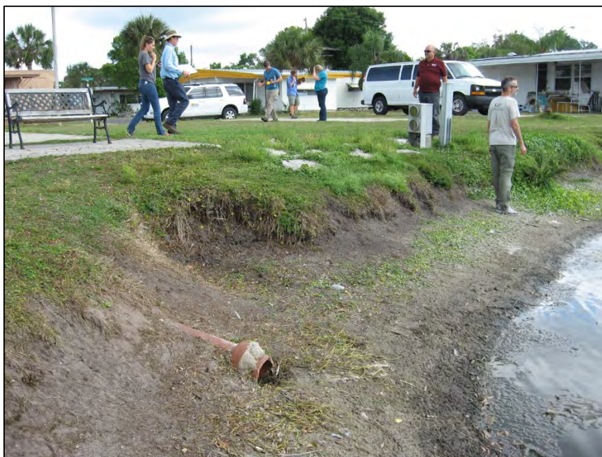
Figure 8. Site C – Boulevard Estates Mobile Home Park – Pond margin with pet and bird feces, as well as numerous pipes. A sewage odor was detected at the pond.
