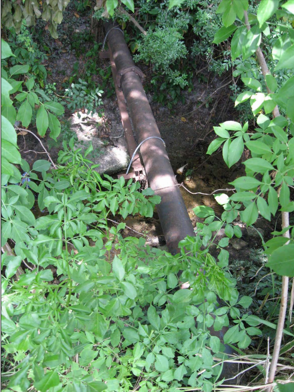
Figure 19. Site F – Alcove Park Mobile Home Park – Ductile iron sanitary sewer pipe crossing Alligator Creek. Pipe needs to be inspected to determine if it is properly installed, supported and restrained.
