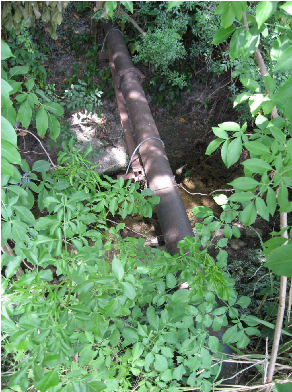
Figure 11. Site F – Alcove Park Mobile Home Park – Ductile iron sanitary sewer pipe crossing Alligator Creek. Pipe needs to be inspected to determine if it is properly installed, supported and restrained.
