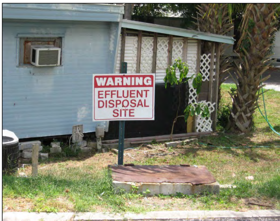
Figure 6. Site A – Southern Comfort Mobile Home Park – Effluent Disposal System. Treated wastewater is pumped up hill to higher areas of the park where it is allowed to infiltrate into the ground.
