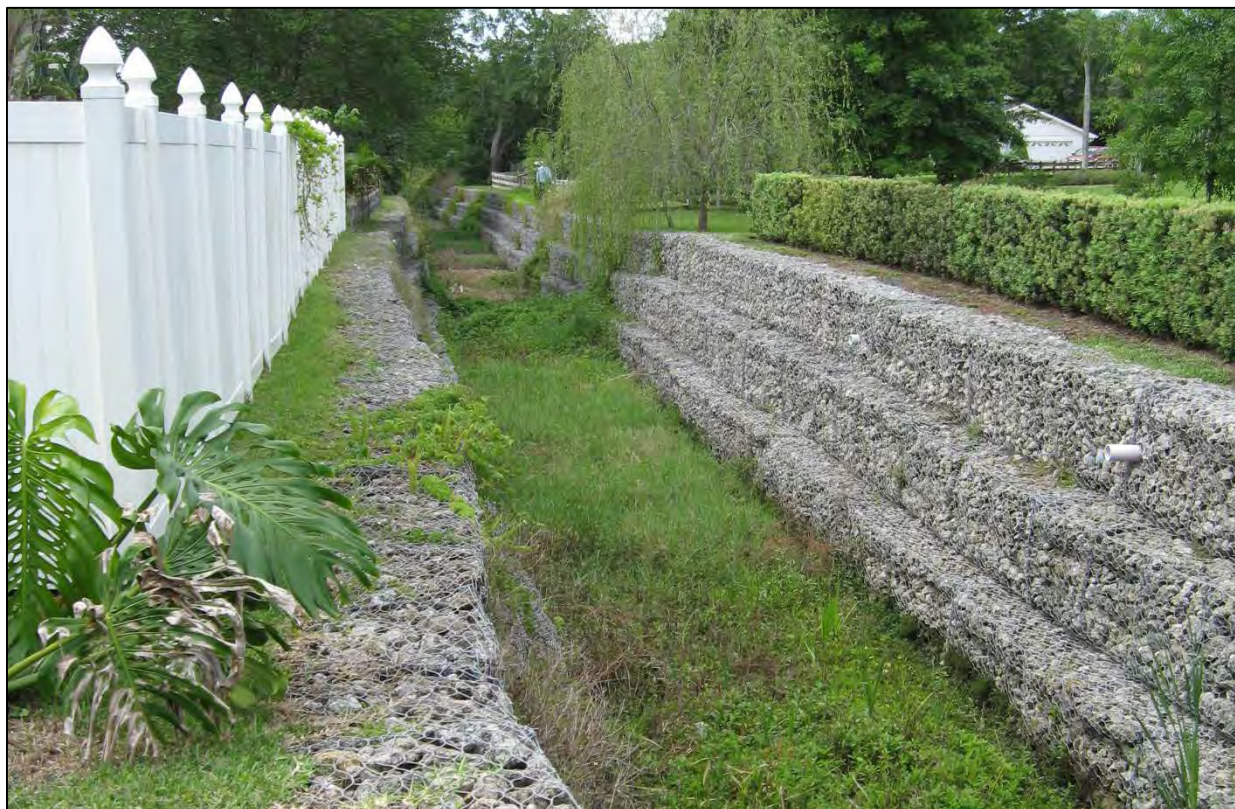
Figure 28. Site P – Coachman Ridge – showing the gabion system and lack of marginal vegetation along Channel F of Alligator Creek.
