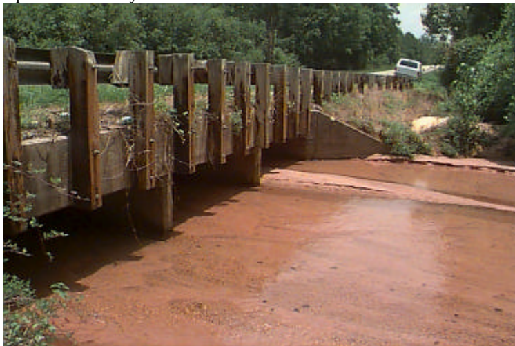
Moore Creek CR 197 – note sediment filled stream channel and resultant lack of capacity to accommodate floodwaters
