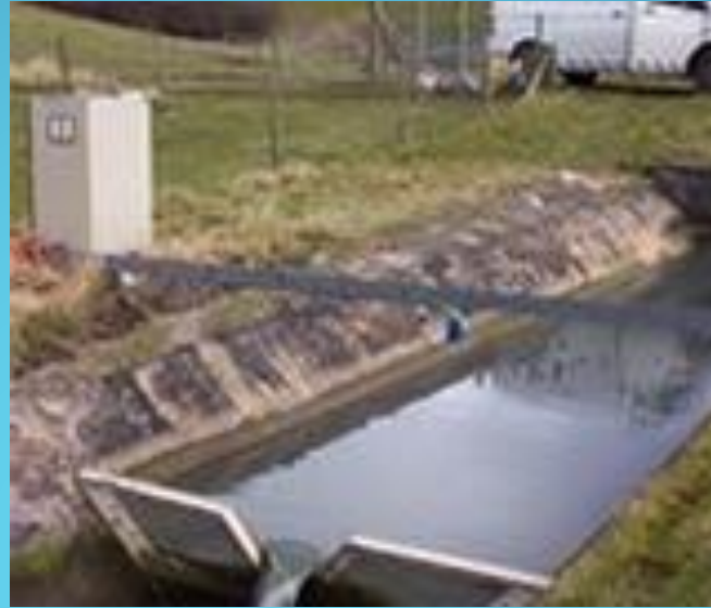
Typical V-Notch Weir installed in a concrete-lined trapezoidal channel
