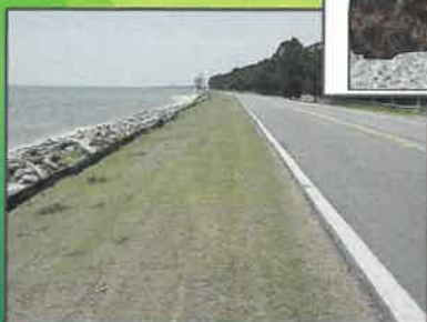
Left: The shoulder of Highway 98, over 8 months after the application, is still stabilized and has held up to the extreme weather conditions of the Florida coast.
