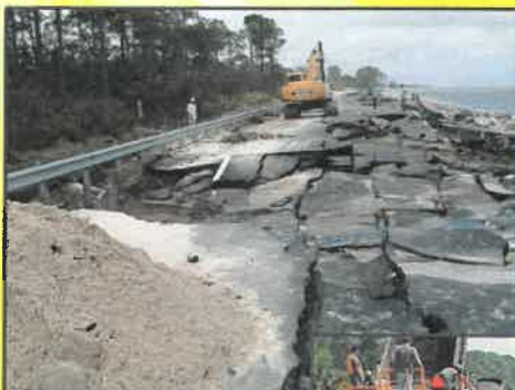
Above: The movement of the highly erosive beach sands caused the roadway to collapse, in some places across the entire width of the two lane road.
