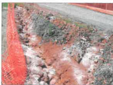
Figure 38. Eroding gully on a construction site
