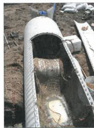
Figure 20. Split pipe with polymer blocks
