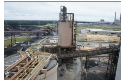
Unit 4 Bottom Ash Dewatering Bin (foreground) Unit 5 Fly Ash Silo and Dewatering Bins (background)
