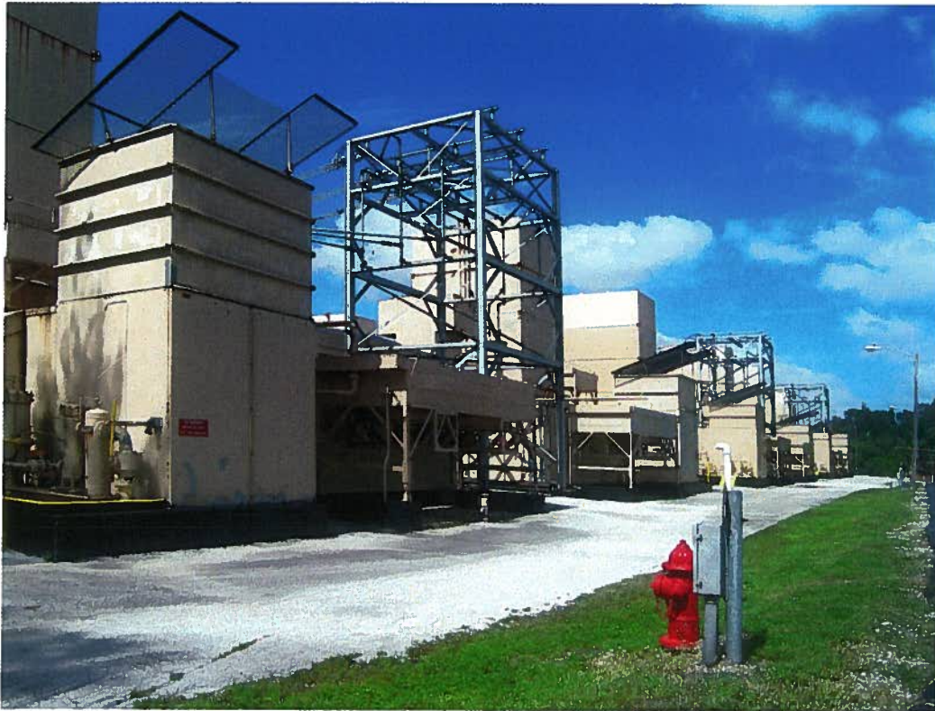
Figure 6. View west of Gas Turbine 2.
