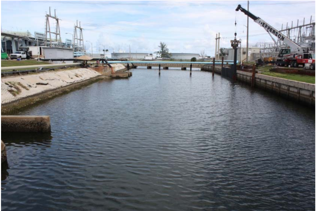
Figure 10.7.1-3. Plant discharge structures and discharge canal
