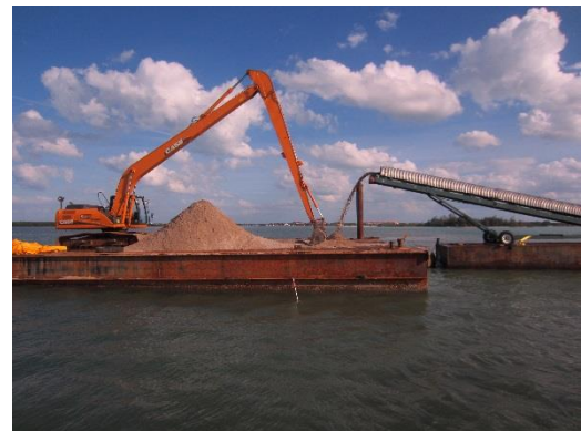
Photo 4-1. Fill conveyor loading placement barge
