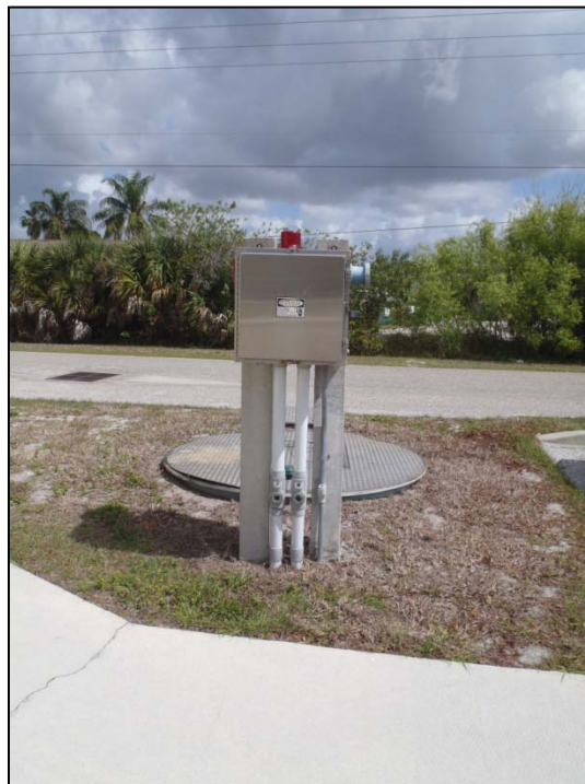
Suncoast Worship Center 881 S. River Road; No Emergency Signage
