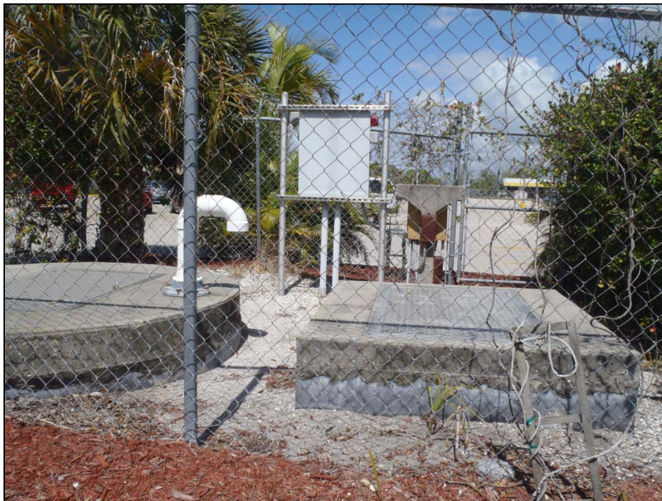
Englewood Center 200 S. Indiana Ave @ Palm Grove Avenue South end of shopping center; No Emergency Signage
