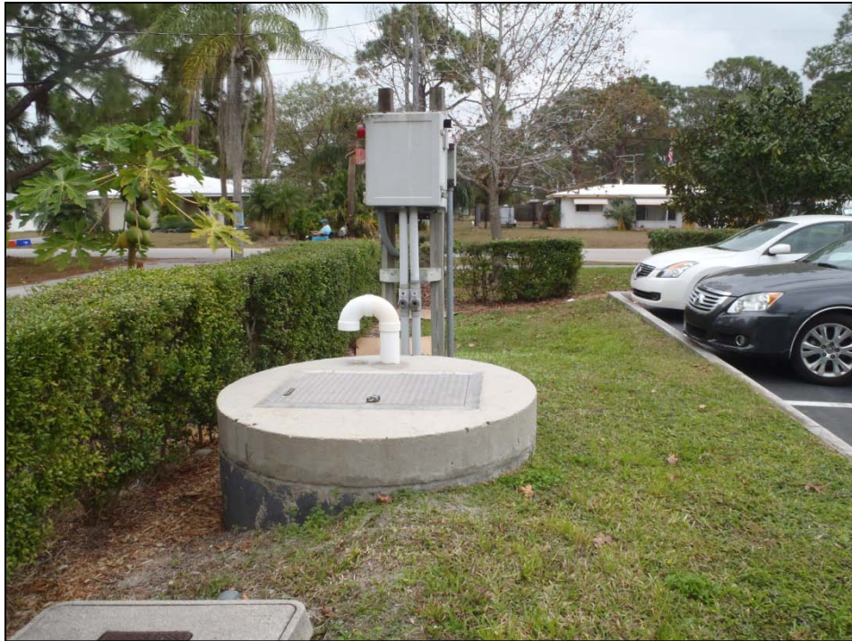
Figure B.5. Private Lift Station P-66.
