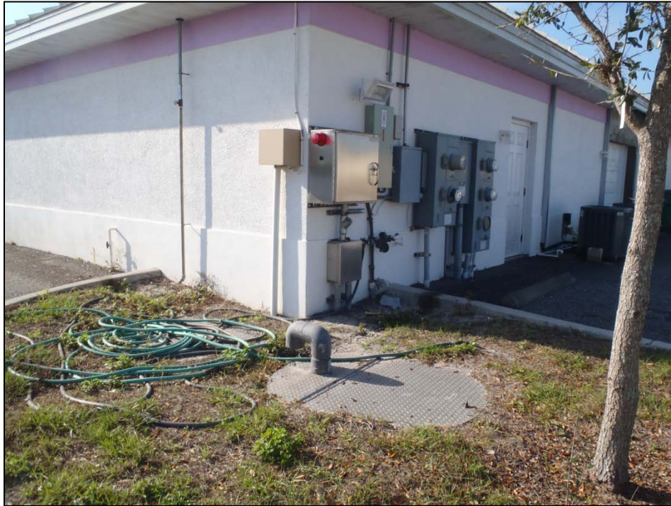
Storage Units 916 S. River Rd.; No Emergency Signage
