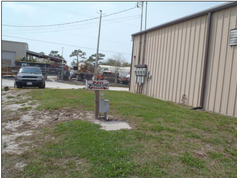
Jones Fogelman Pool & Spa Services 858 S. River Rd.; No Emergency Signage
