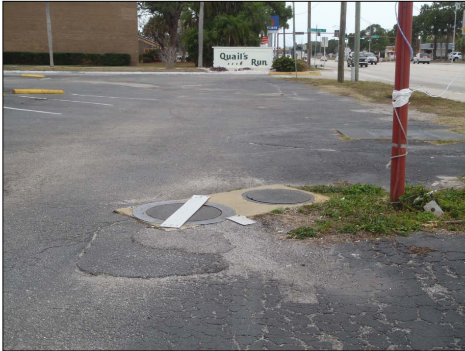
Englewood Bowl, 299 S. Indiana Avenue In front parking lot; No Emergency Signage or Alarm
