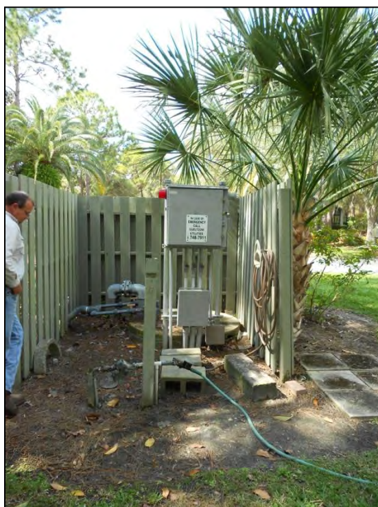
Figure 44. Gasparilla Condominium – Private Lift Station.
