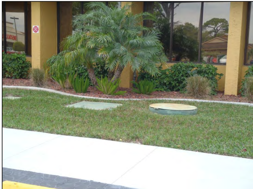
Figure 4. Private Lift Station – Provision Eye Center.
