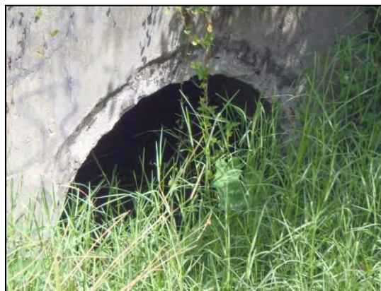
Figure 103. Stormwater Pipe from DP38-184 to Vault.
