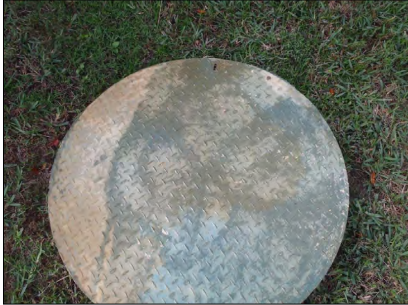
Figure 3. Private Lift Station – Provision Eye Center
