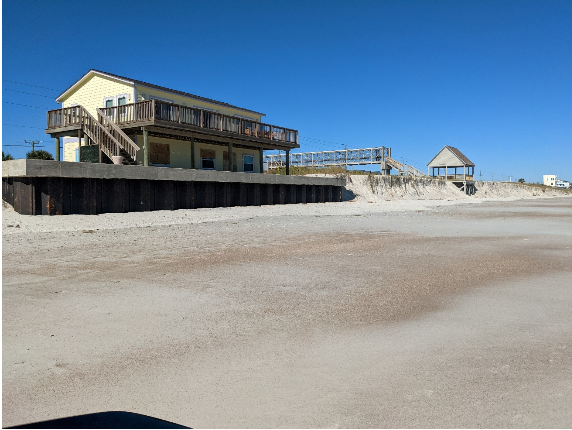
Figure 4: Photo facing northwest just south of Carcaba Road (R-114) showing post-storm dune scarping, exposure of pre-existing seawalls, and undermining of beach access structures. The large beach access structure in the background cross SR A1a and connects to the Villages of Vilano. November 16, 2021
