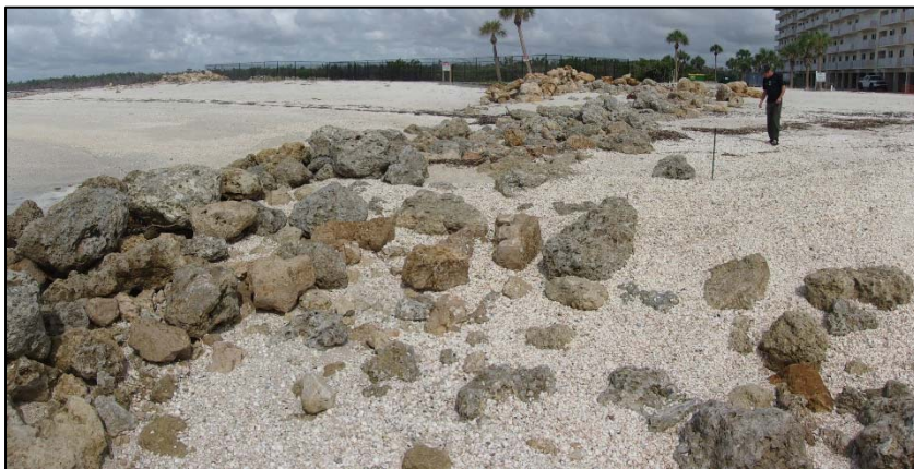
Figure 6: South groin (photo - 9/26/2023), 1 year after Hurricane Ian. At top: seaward end. At left: central stem and landward end.
