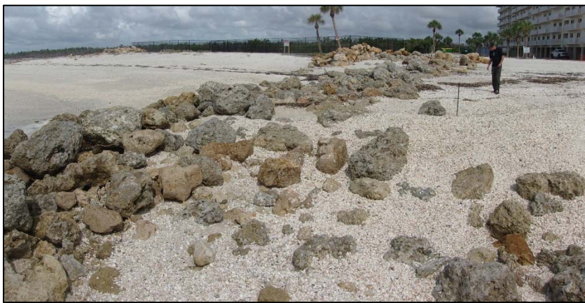
Figure 2: South groin (photo - 9/26/2023), 1 year after Hurricane Ian. At top: seaward end. At left: central stem and landward end.
