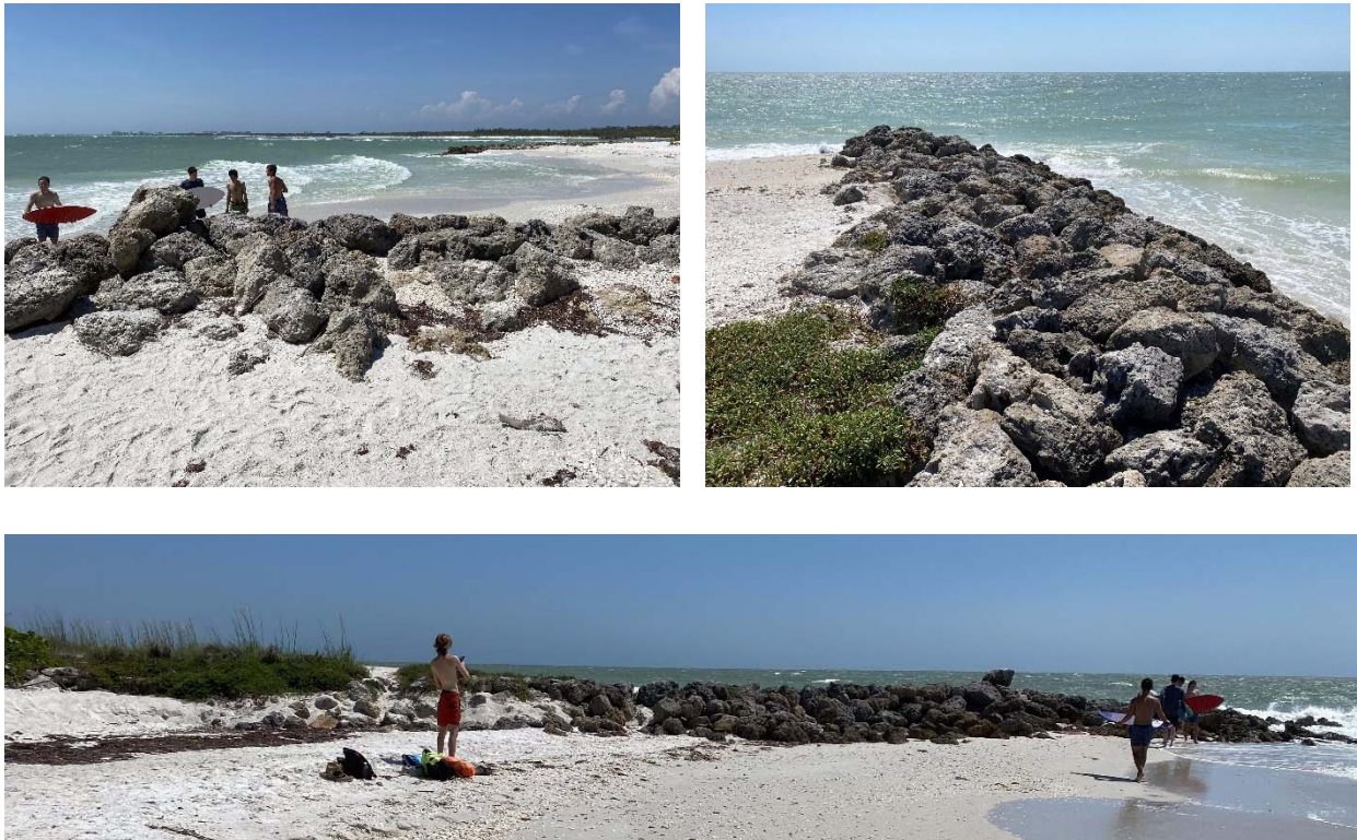
Figure 5: Left – South groin. Right – North groin. Lower – South groin. Pre- Hurricane Ian; 4 May 2021. Photos by Vadim Alymov (Coastal Engineering Consultants, Inc.).
