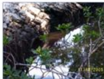
Existing Partially-functional 60 Inch Culvert
